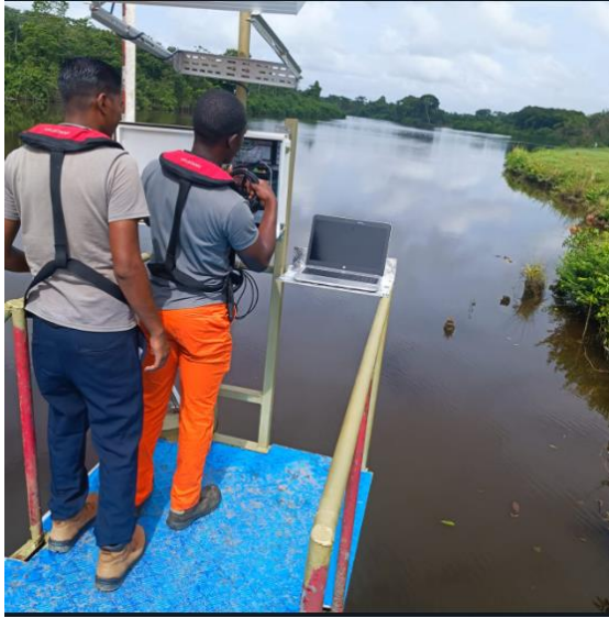
Figure 6: Instalment and configuring of new tide station at Traymore Port, Cottica River.
