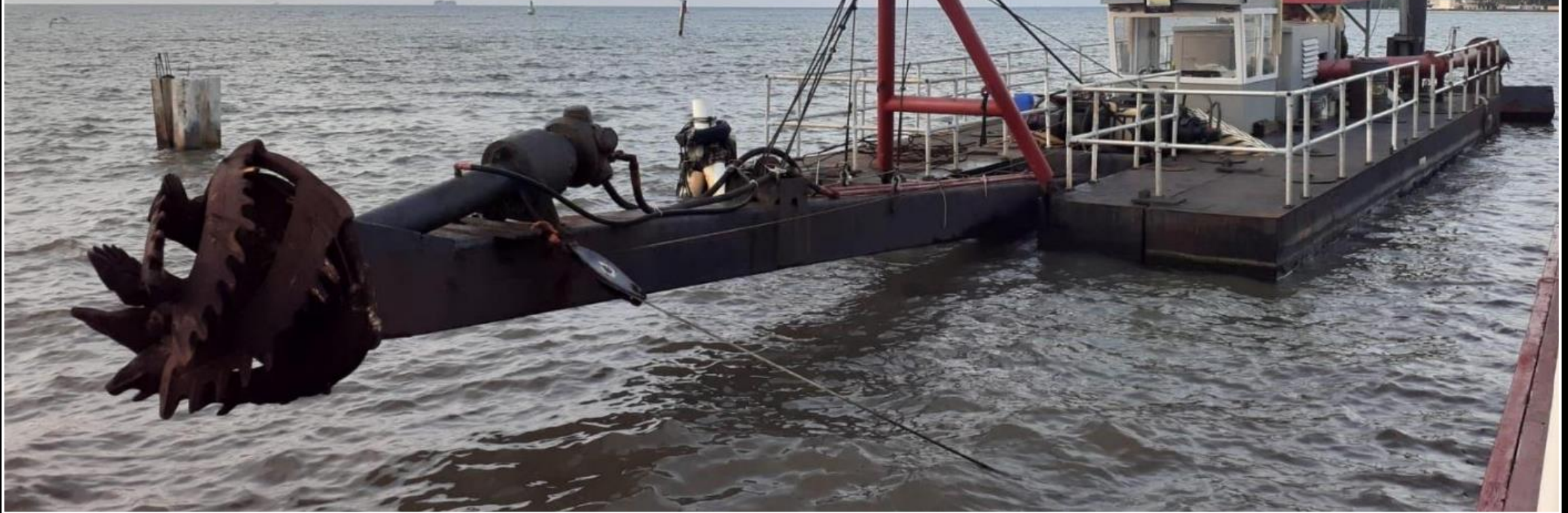
Maintenance dredging of Haulover Creek, safe navigation for tender vessels servicing cruise ship calls.
