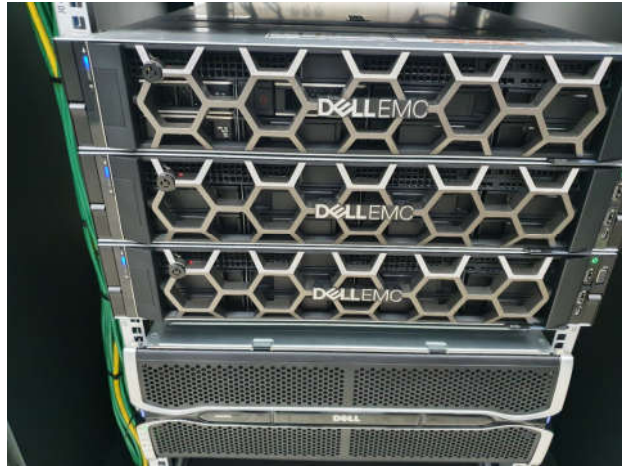
Figure 15. New server communication infrastructure
