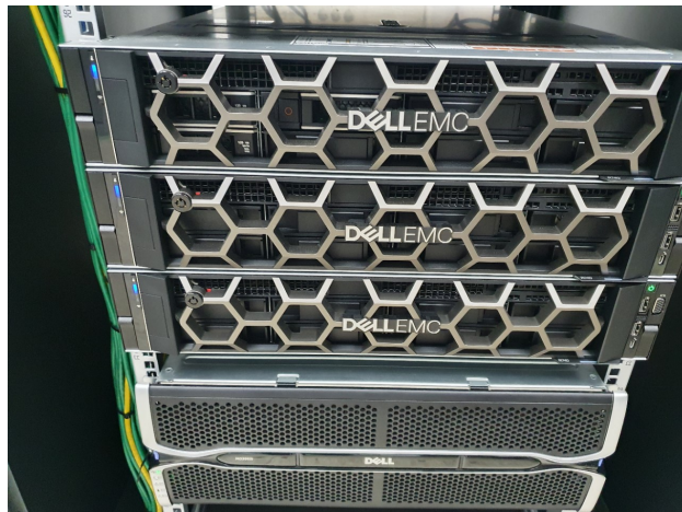
Figure 26. Server infrastructure in the CHI Data Centre
