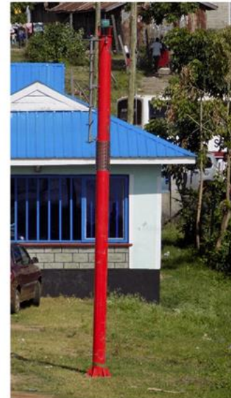
Pic 10: LUANDA KOTIENO SOUTH BERTH LIMIT LIGHT
