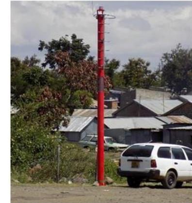
Pic 9: MBITA EAST BERTH LIMIT LIGHT
