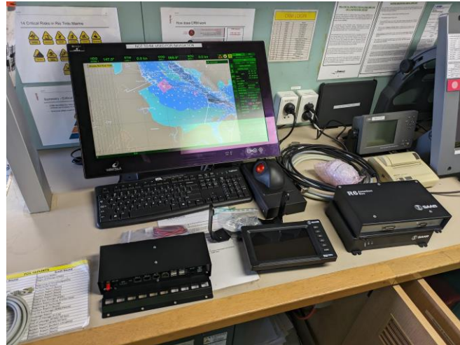
Figure 1: Installation of the VDES hardware that is used to receive S-124 data onboard ships.
